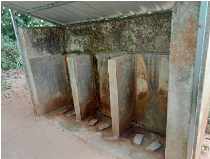
Figure 15 Boys urinals also have no privacy wall
