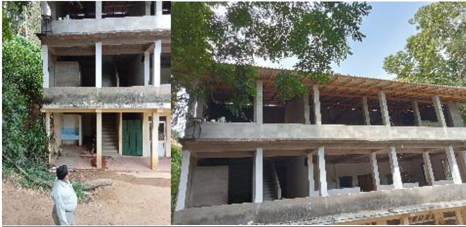
Figure 16 Unfinished building, Soil not established, no drainage, danger in erosion
