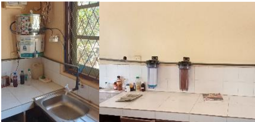
Figure 5 Water Filters for Pipe water
